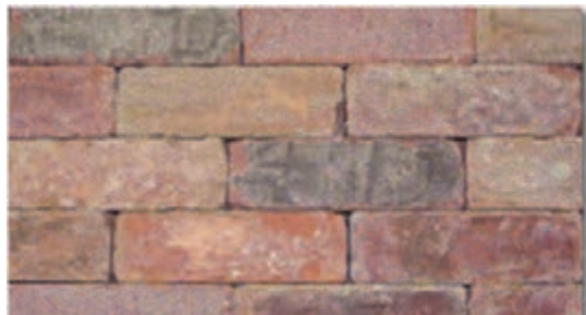
No Mortar Joint (Dry-Stacked)
